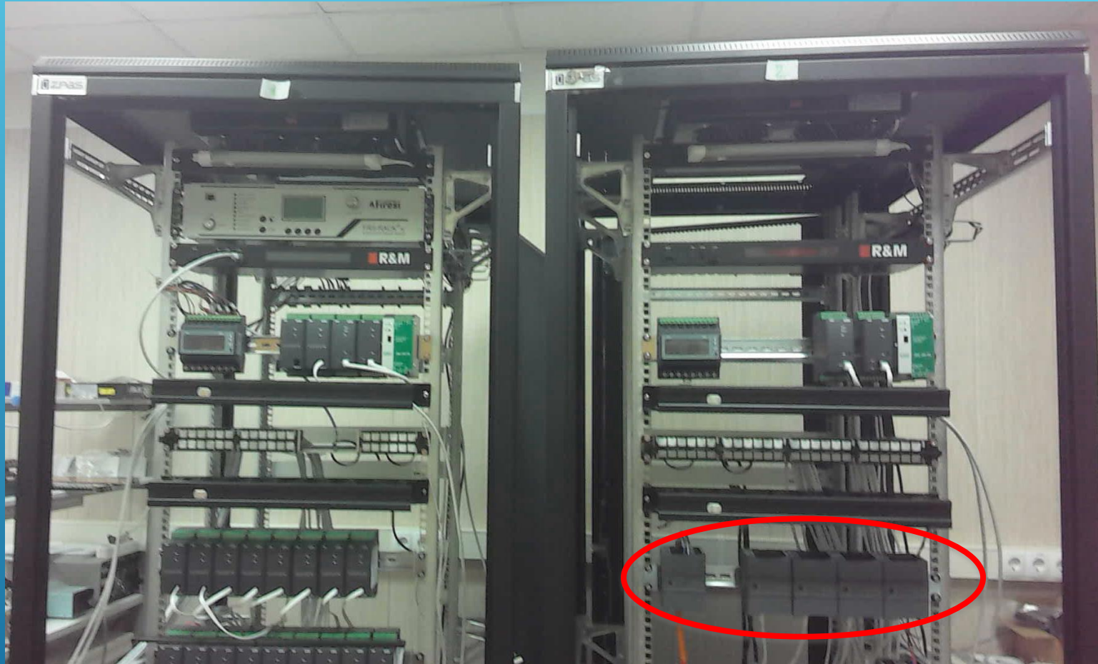
Master & Slave Racks Slow Control Run Start System BM@N
